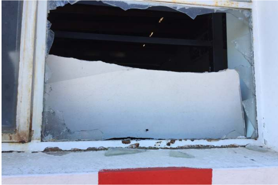
Photograph 13: Main Building, interior, southwest toilet block, loose panels, fibre cement sheeting, asbestos (assumed)
