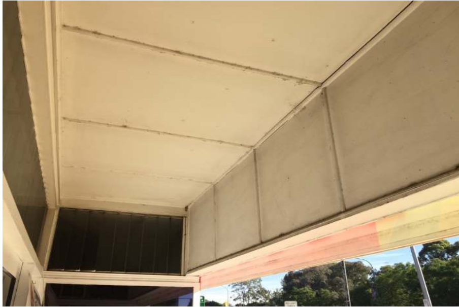
Photograph 5: Main Building, exterior, northern entrance, ceiling and fascia lining, fibre cement sheeting, asbestos detected by analysis.
