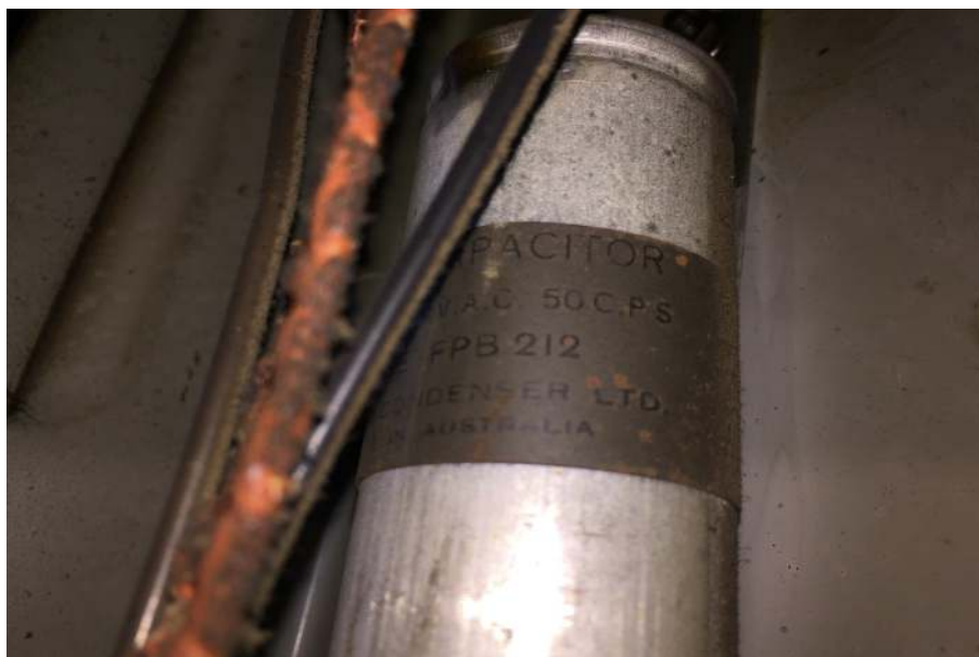
Photograph 55: Main Building, interior, warehouse area, northwest corner, metal capacitor (DUCON, Type FPB 212) insulating oil, PCB (assumed)
