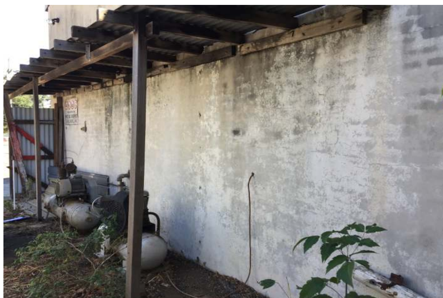
Photograph 22: Main Building, exterior, east, typical wall lining, white paint, lead paint (>0.1% lead w/w).
