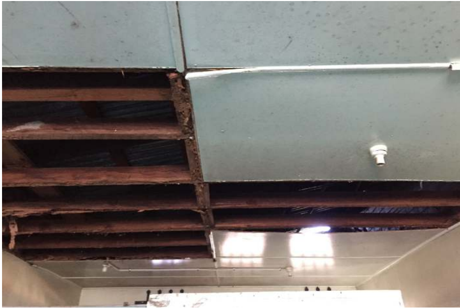
Photograph 19: Main Building, interior, southwest toilet block, ceiling, fibre cement sheeting , asbestos detected by analysis
