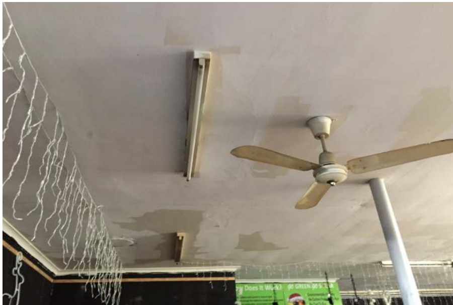
Photograph 40: Main Building, throughout, fans, capacitors, insulating oil, PCB (assumed).
