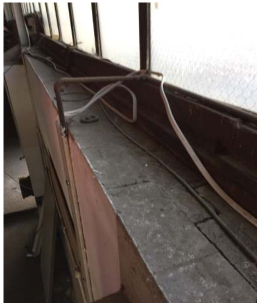
Photograph 36: Main Building, interior, main warehouse, southern end, ledge below windows of saw-tooth roof, settled dust/debris, elevated lead (61 mg/m 2 )
