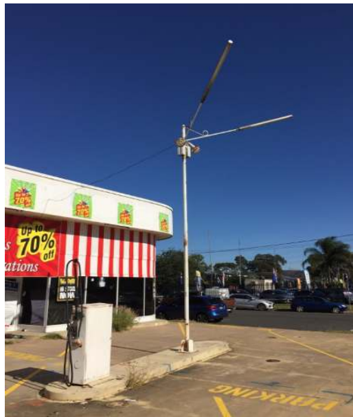
Photograph 14: Main Building, exterior, north, light pole, fluorescent light fittings, capacitors/ballasts, insulating oil, PCB (assumed).
