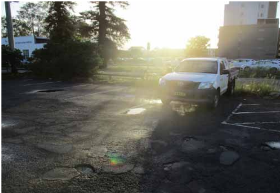
Photo 6 - Bitumen carpark showing cracked broken areas
