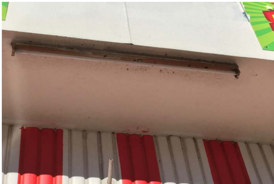
Photograph 4: Main Building, exterior, north and west eaves, fluorescent light fittings (approx. 5), capacitors/ballasts, insulating oil, PCB (assumed).
