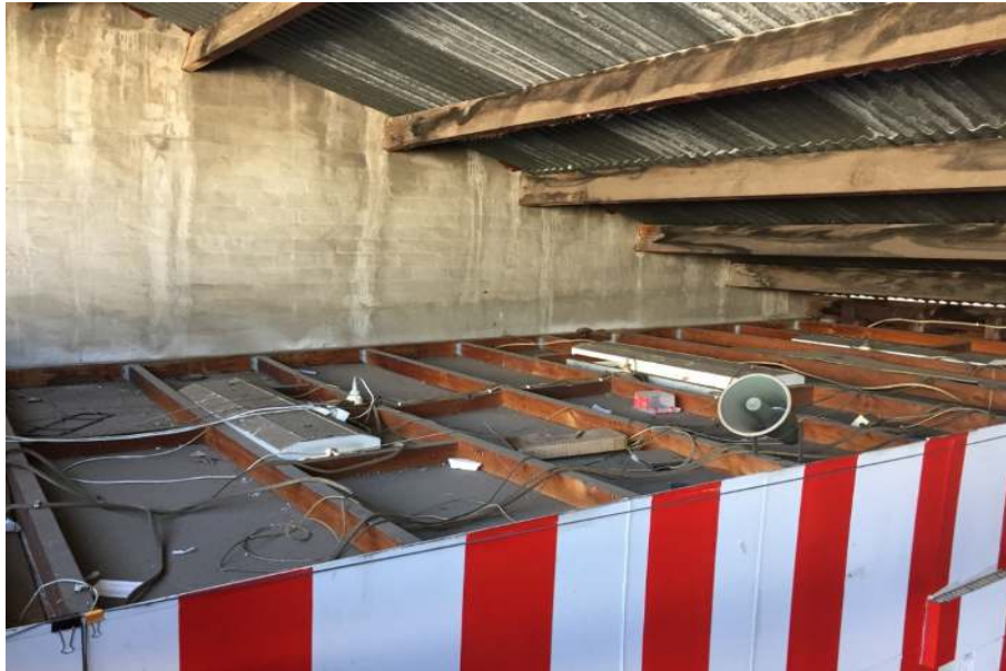
Photograph 35: Main Building, interior, main warehouse, office area, top of ceiling, settled dust/debris, elevated lead (42 mg/m 2 )
