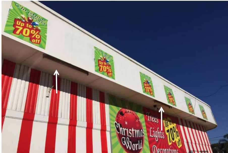
Photograph 3: Main Building, exterior, north and west, eave lining to showroom, fibre cement sheeting, asbestos (assumed)
