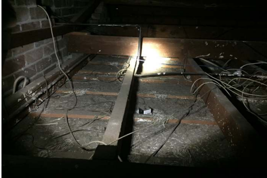
Photograph 41: Main Building, interior, northern entrance, ceiling cavity, settled dust/debris, elevated lead (120 mg/m 2 )
