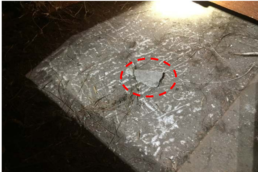
Photograph 42: Main Building, interior, northern entrance, ceiling cavity, fibre cement sheeting debris, asbestos detected by analysis.
