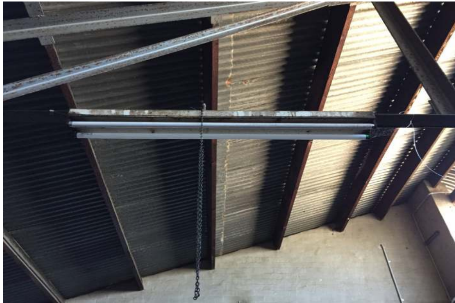
Photograph 39: Main Building, interior throughout, fluorescent light fittings in general (approx. 50), capacitors/ballasts, insulating oil, PCB (assumed).
