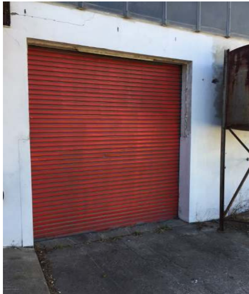
Photograph 24: Main Building, exterior, south, roller door, red paint, lead paint (>0.1% lead w/w).
