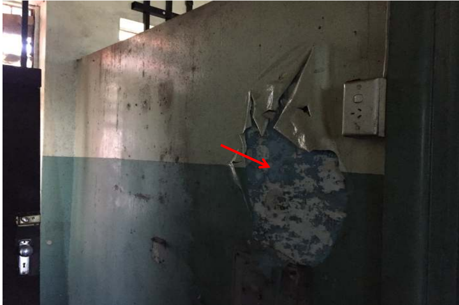
Photograph 47: Main Building, interior, southwestern toilets, typical wall, underlying blue paint, lead paint (>0.1% lead w/w)
