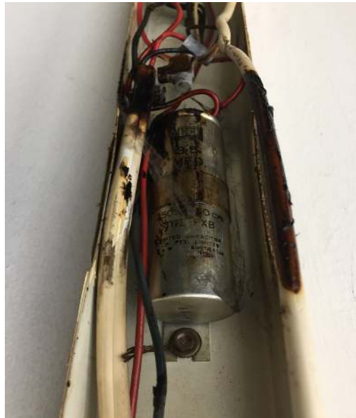
Photograph 54: Main Building, interior, northern shopfront, metal capacitor (UCC, 3.5 MFD 250v AC 50 CP3, TYPE PBX) insulating oil, PCB (assumed)
