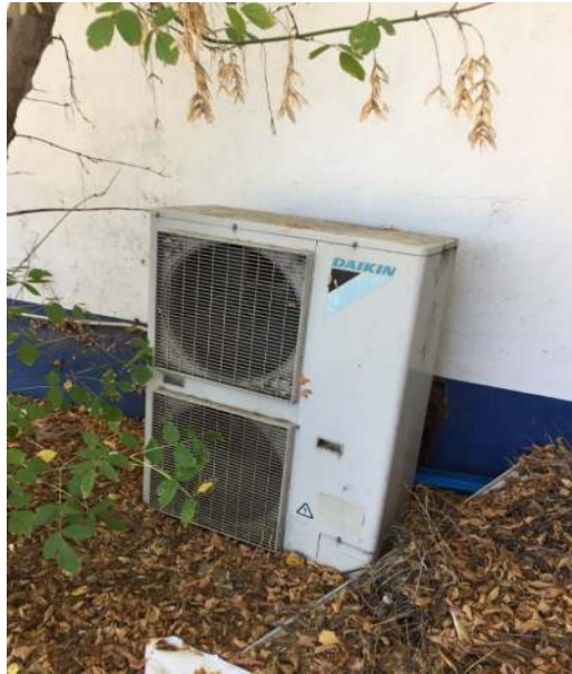
Photograph 44: Main Building, exterior, eastern side, air conditioning unit, internal insulation, SMF (assumed).
