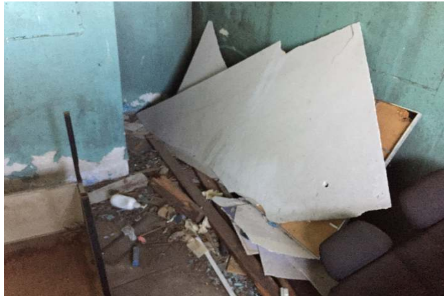
Photograph 58: Main Building, interior, southwest toilet block throughout, damaged sheeting and associated dust/debris, fibre cement sheeting, asbestos detected by analysis
