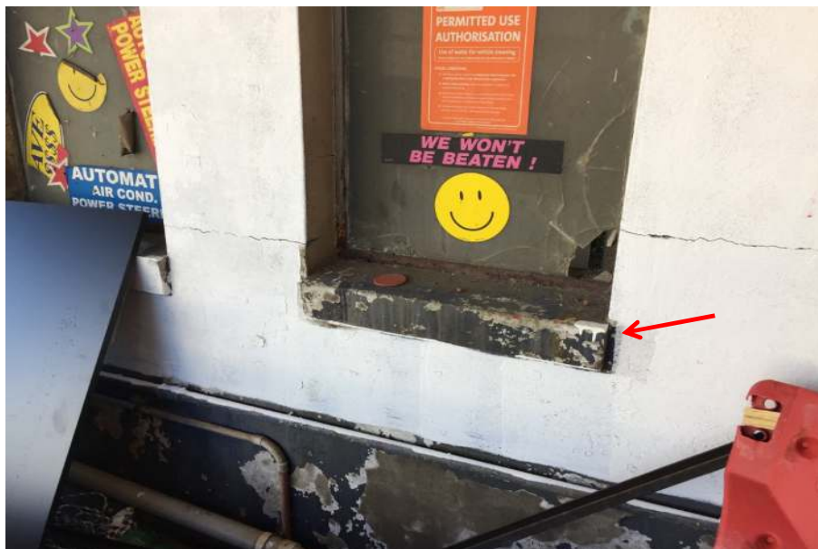
Photograph 21: Main Building, exterior, southwest, toilet block, window sill, blue paint, lead paint (>0.1% lead w/w).
