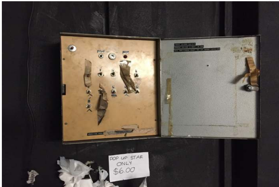
Photograph 30: Main Building, interior, northern entrance area, alarm panel, internal components, unknown (inaccessible).
