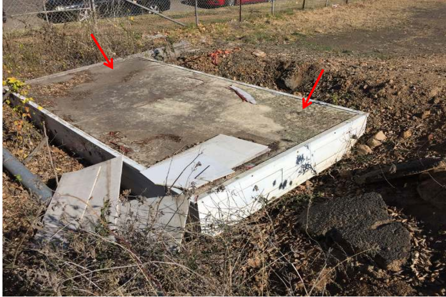
Photograph 53: Exterior grounds, southern end of site, demolished signage, internal fluorescent light fittings (if present), capacitors/ballasts, insulating oil, PCB (assumed)
