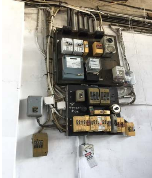
Photograph 33: Main Building, interior, main warehouse, northeast corner, black electrical boards (2 units), asbestos (assumed).
