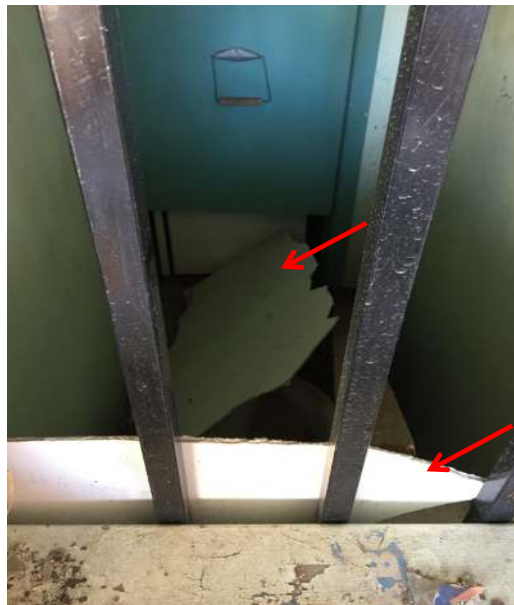
Photograph 20: Main Building, interior, southwest toilet block throughout, damaged sheeting and associated dust/debris, fibre cement sheeting, asbestos (assumed)
