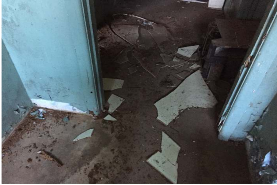
Photograph 57: Main Building, interior, southwest toilet block throughout, damaged sheeting and associated dust/debris, fibre cement sheeting, asbestos detected by analysis
