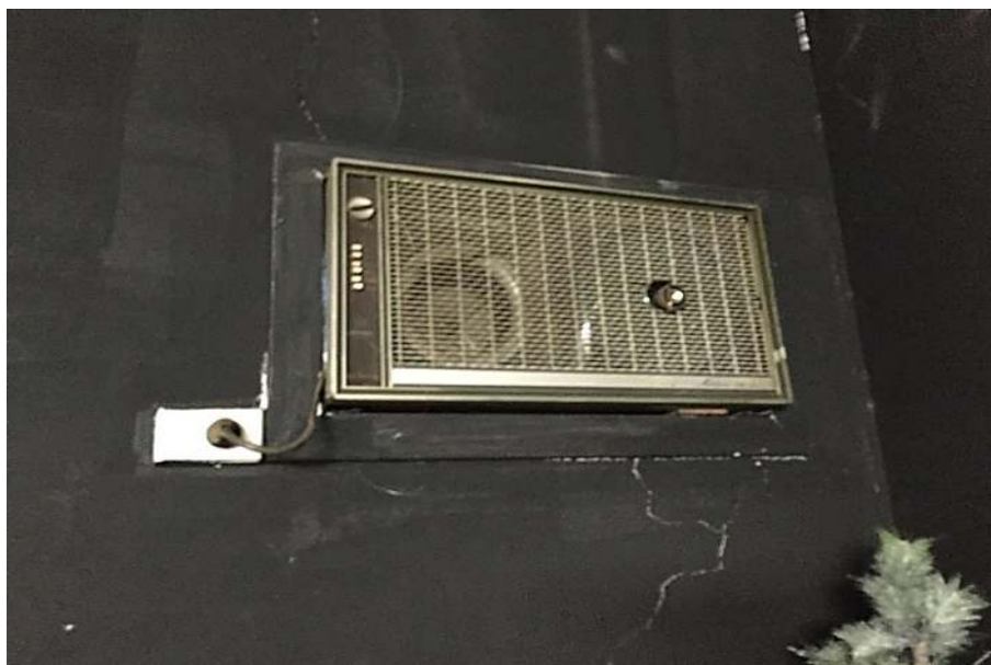
Photograph 38: Main Building, interior, northwest corner, air conditioning unit, internal insulation material(s), SMF (assumed).
