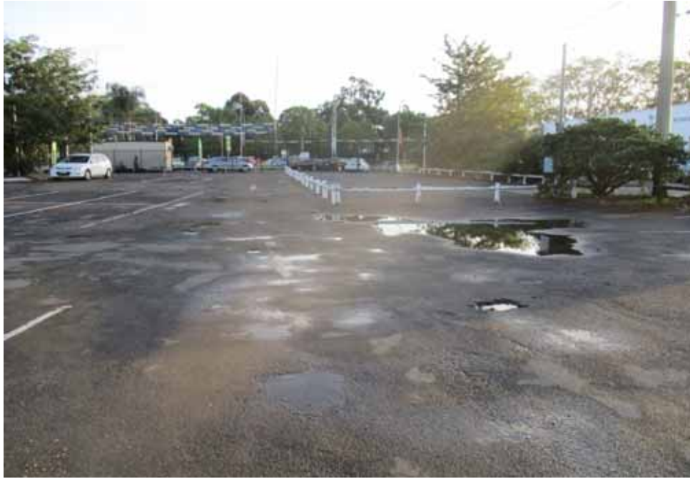
Photo 5 - bitumen carpark with dips and ponding
