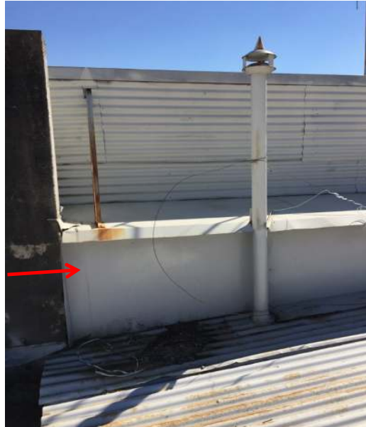
Photograph 25: Main Building, exterior, main roof, sections of parapet wall lining, fibre cement sheeting, asbestos detected by analysis
