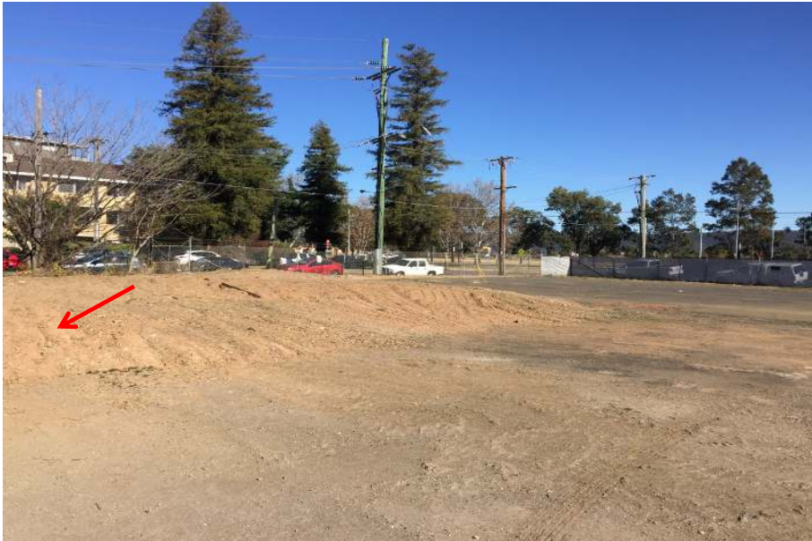
Photograph 52: Exterior grounds, southern end of site, ground surfaces, fill, fibre cement sheeting debris, asbestos detected by analysis
